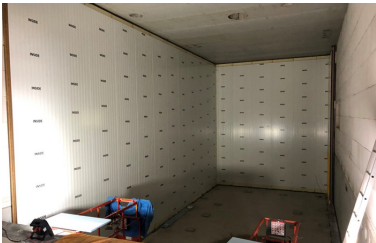
Insulation of the climatic test bench
